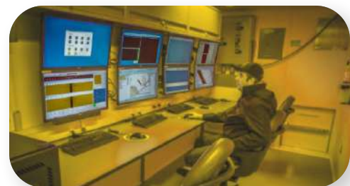
Klein custom designed control room in ISO container
