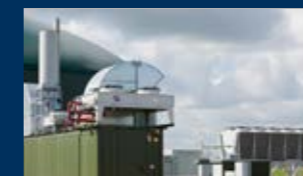
Installation biogaz ElectraTherm Trechwitz, Allemagne
