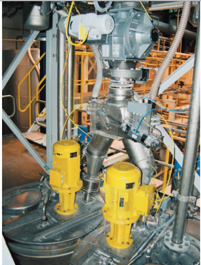
YTRON-Y ByPass in the Brewing Industry Application: Suspending of Diatomaceous Earth CO 2 inerting for a Continuous Discharge of the Product.
