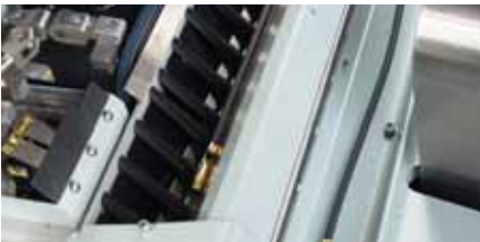
Optional Continuity Tester with Sort of Failed Wires
