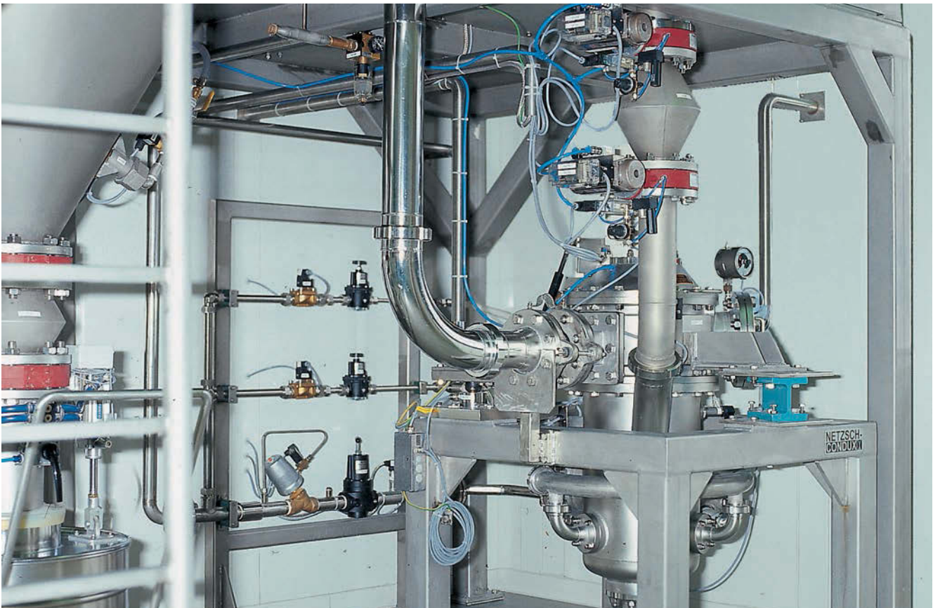
Installation with Fluidized Bed Jet Mill CGS 32 in „Pharma design“
