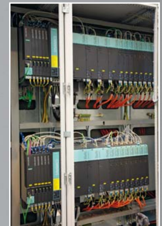
■ Drive control unit SIEMENS
