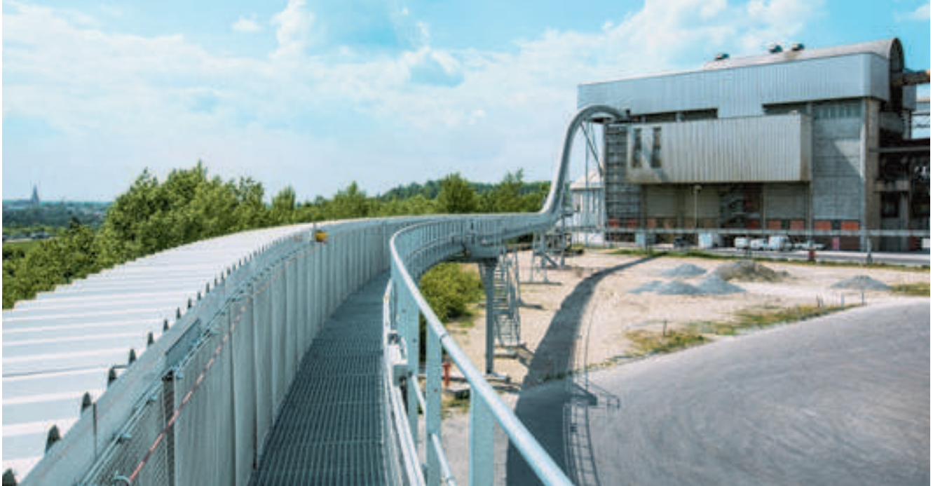
BEUMER pipe conveyor
