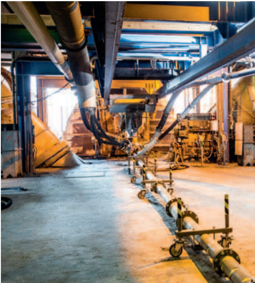
Pneumatic conveying line to the main burner
