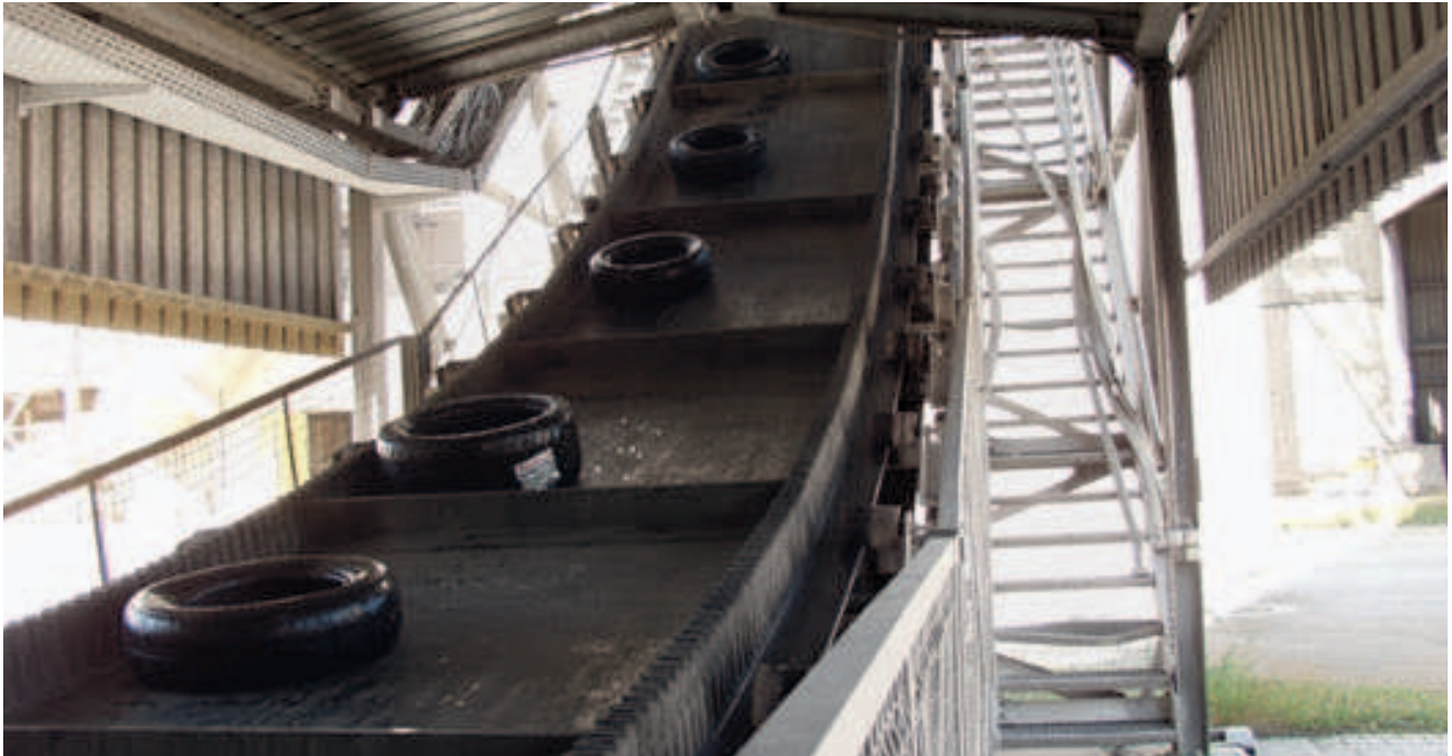
Steep incline conveyor lifts total tires from the ground level to the point of feeding at the preheater.
