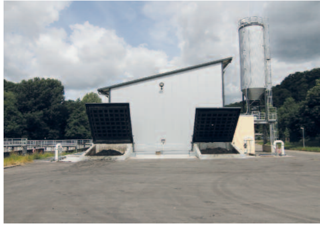
Sludge bunker and dry material silo
