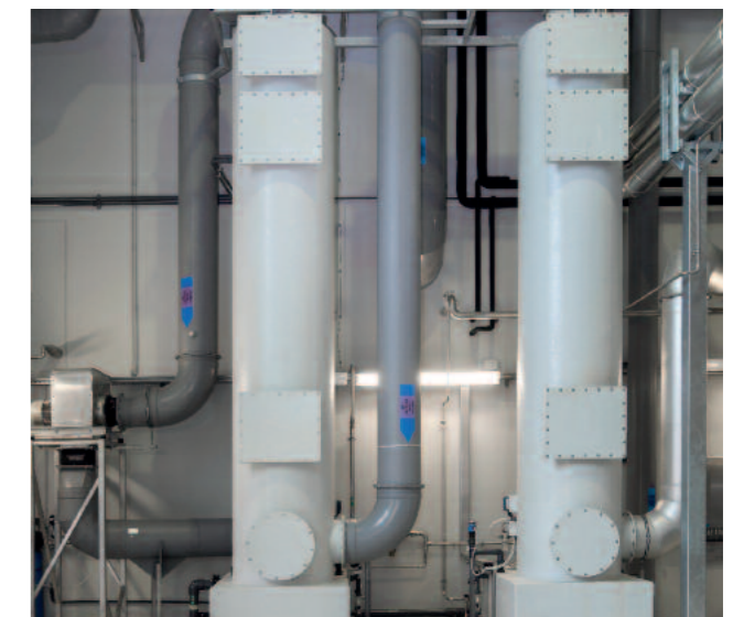
Two stage scrubber for odor control
