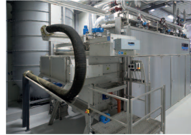
Sludge feeding with HUBER extruder unit (pelletizer)
