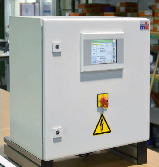
Control cabinet with operator panel on which minor program changes can be made directly
