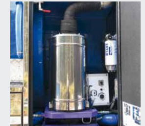
Water heater "Hot-Box"
