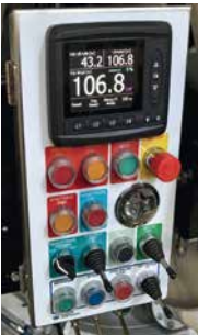
Rear control panel with IOAN display
