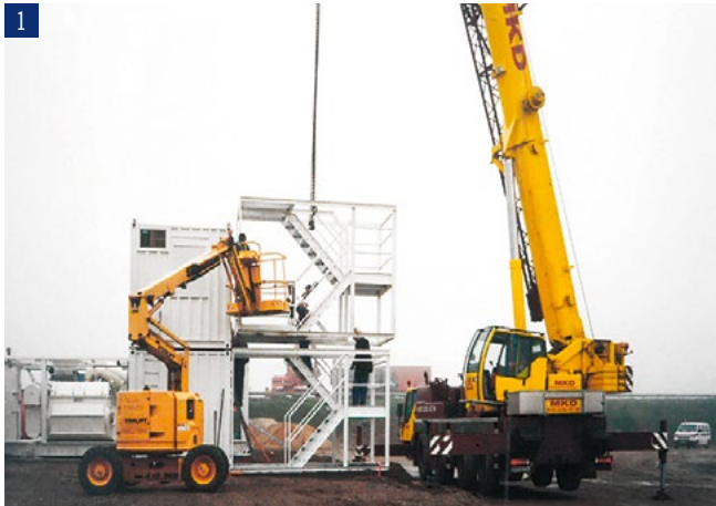
1 Installation of the chemical storage and control room containers on leveled ground
