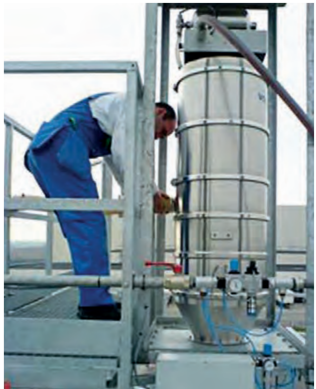
Vacuum conveyors in an outdoor installation, for charging silos.
